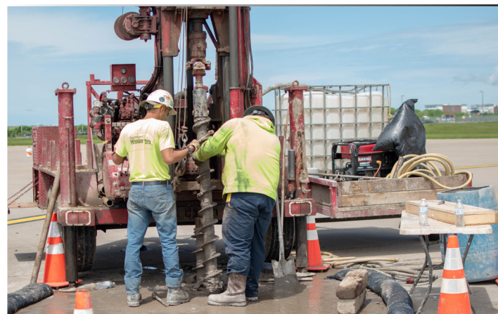
Geotechnical services to determine soil conditions are underway at the construction site of the new terminal between Concourses C and D.
